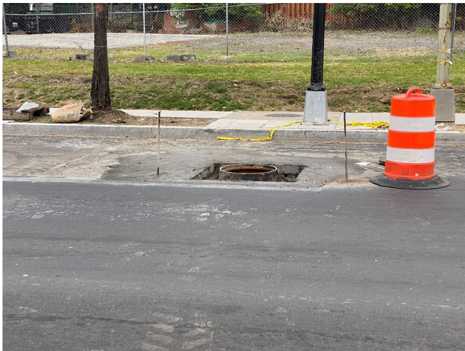
Picture No. 12 – 10/10/2020 – Manhole reset in progress along NY Ave between 3 rd St. and 4 th St. (North view)
