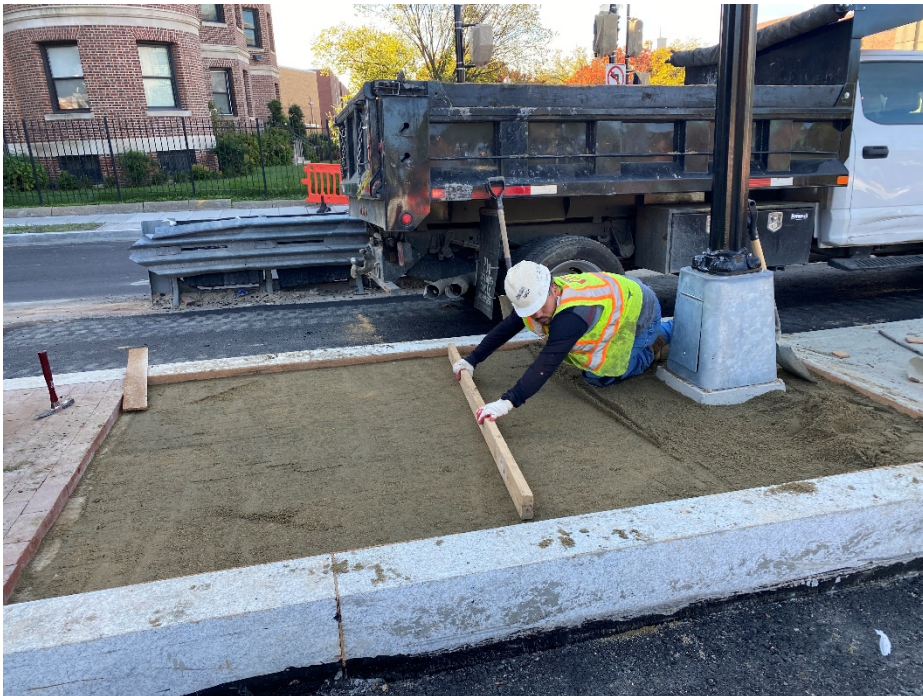
Picture No. 10 – 10/09/2020 – Placement of brick median along NY Ave and NJ Ave intersection (South View)
