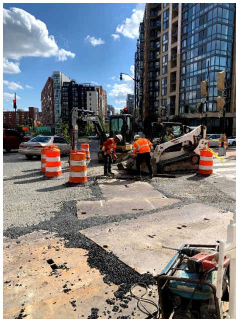
Picture No. 2: 10/05/2020 – Steel plates being placed for the conduit trench at the intersection of NY Ave and 4 th St. (South View)
