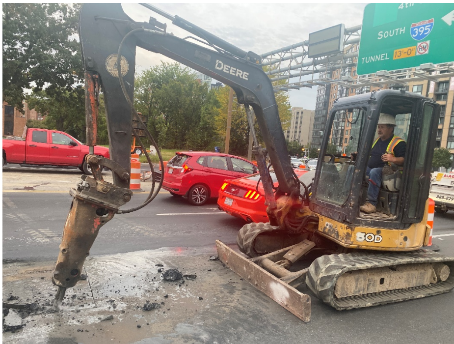
Picture No. 11 – 10/10/2020 – Roadway excavation in progress along NY Ave between 3 rd St. and 4 th St. (Southwest view)
