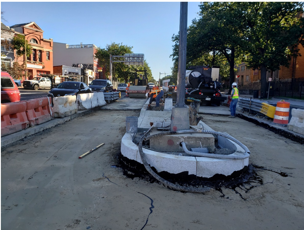
10/08/2020 – Application of tack coat along NY Ave and NJ Ave intersection (East View)
