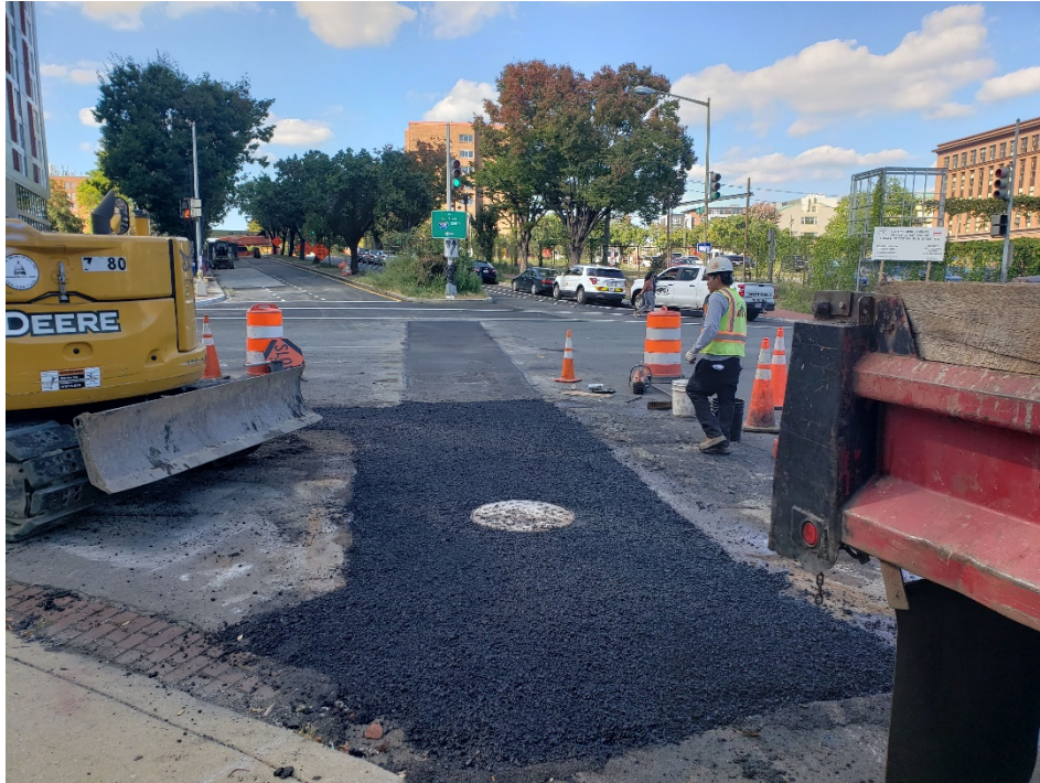
Picture No. 3 – 10/06/2020 – Asphalt placement at the intersection of NJ Ave and H St. (East View)
