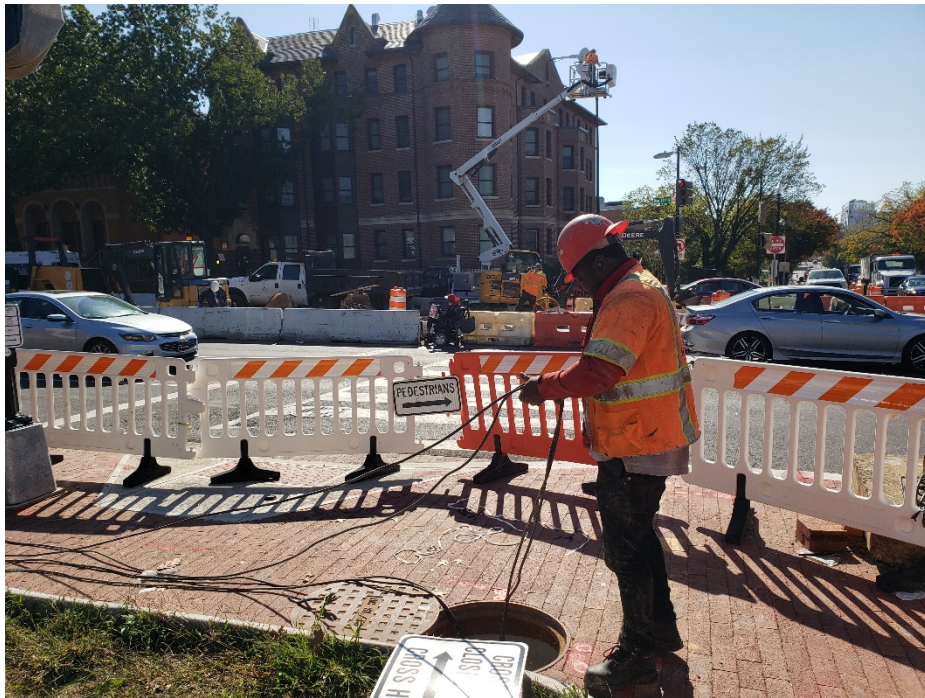
Picture No. 7 – 10/07/2020 – Pulling wires at NY Ave and NJ Ave intersection (North View)
