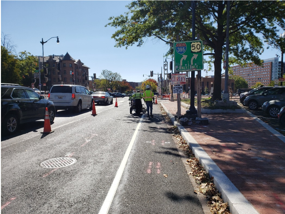
Picture No. 9 – 10/08/2020 – Placement of pavement markings along NJ Ave between N St. and NY Ave (South view)
