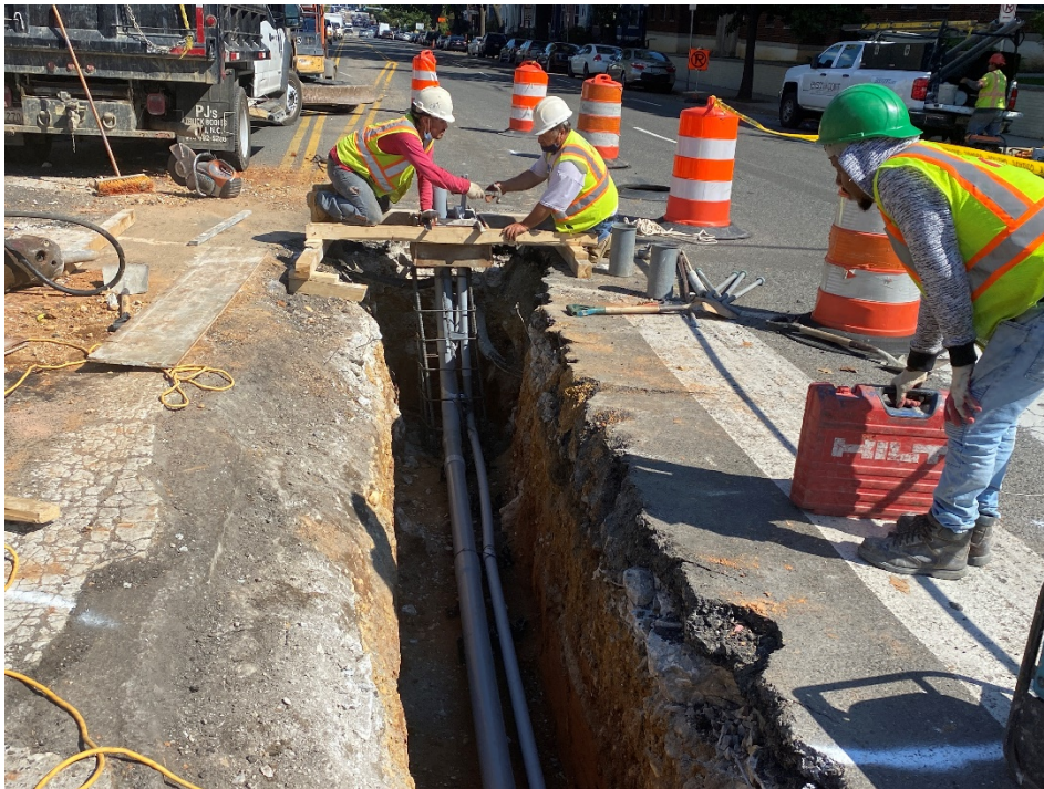
Picture No. 4 – 10/06/2020 – Installation of PVC conduit in the trench near NY Ave and 1 st St. (East View)
