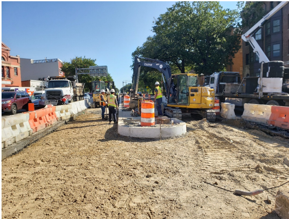
Picture No. 6 – 10/07/2020 – Placement of aggregate base course at NY Ave and NJ Ave intersection (East View)
