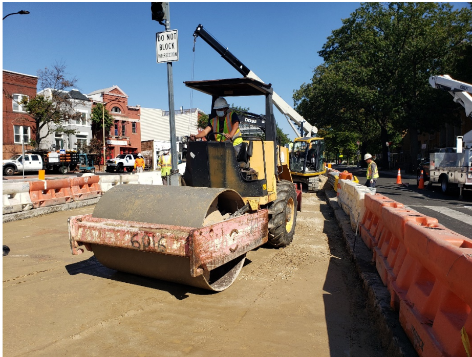
Picture No. 5 – 10/07/2020 – Placement and compaction of aggregate base course at NY Ave and NJ Ave intersection (East View)
