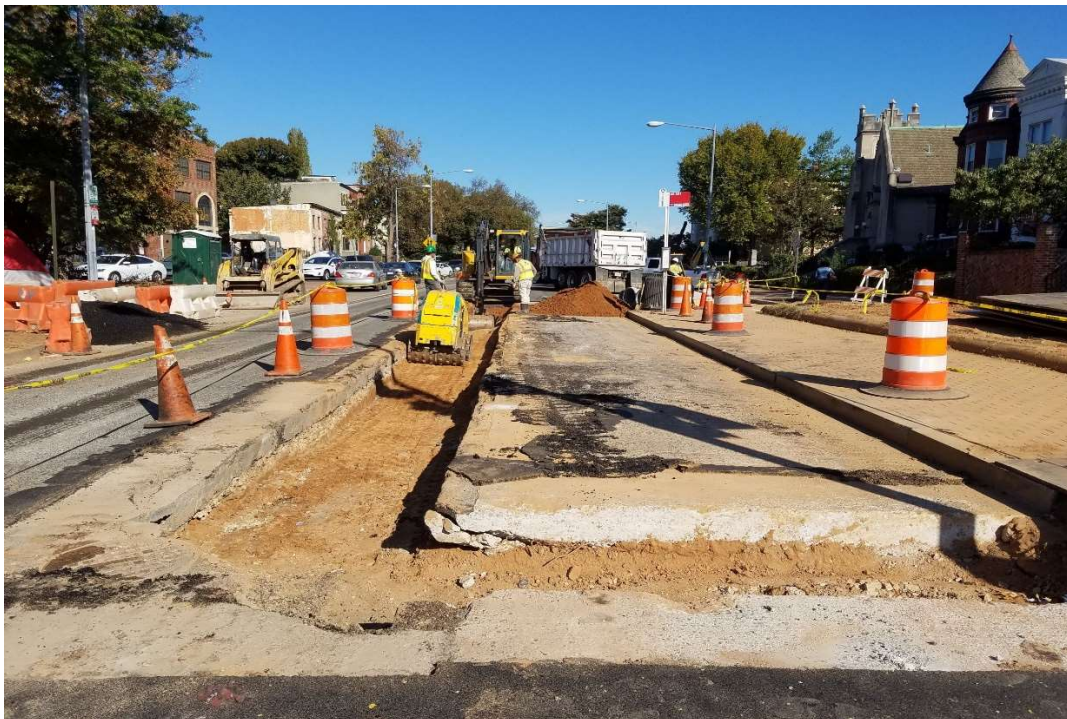
10/15/2019- Soil backfill/compaction for storm pipe installed between MH F-2 & MH F-4 (North View)
