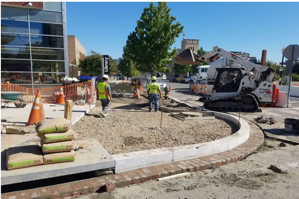
10/14/2019- GAB placement/compaction for SW & WCR at NE corner of NJ & L St. NW. (East View)
