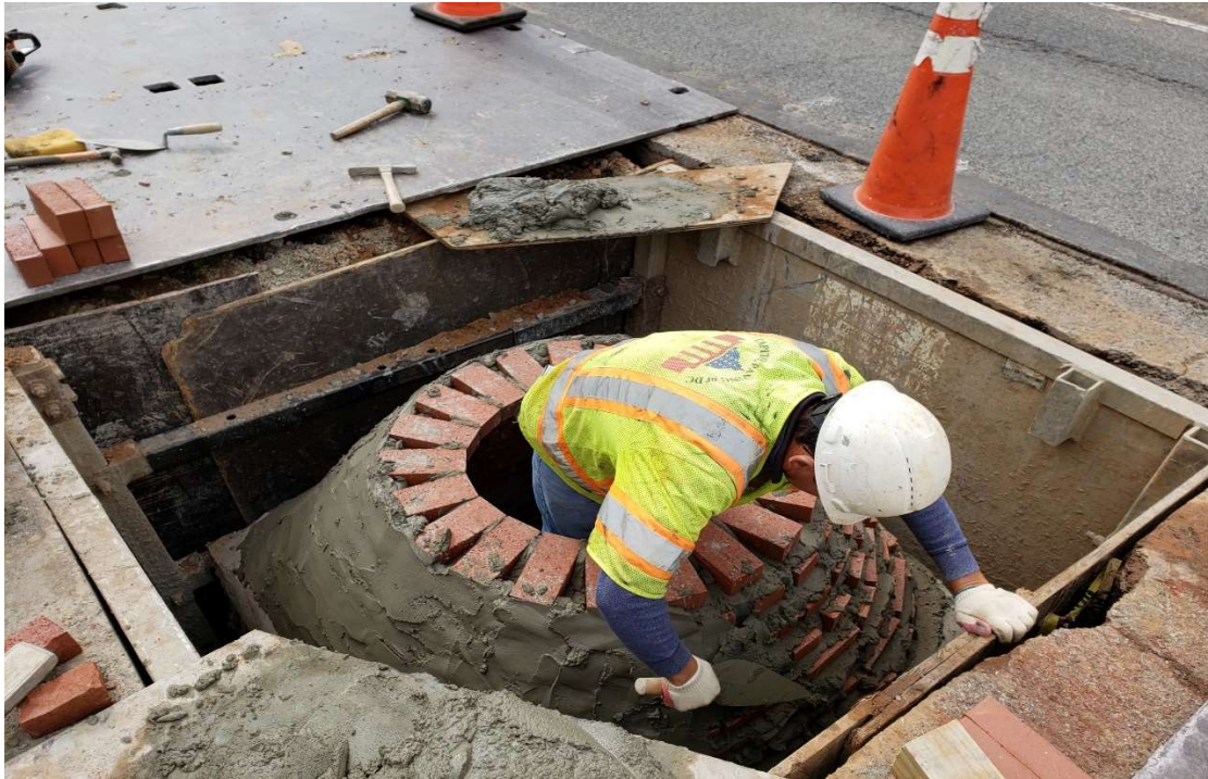
10/17/2019- Installing MH-F4 at NJ Ave. NW between M and Morgan St. NW.
