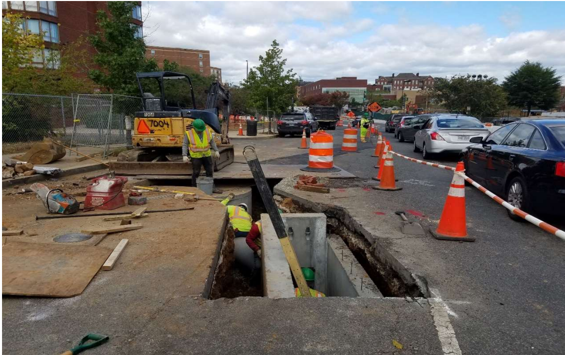
10/17/2019- Installing CB-U1 connection to U1A at NJ & K St. NW (South View)
