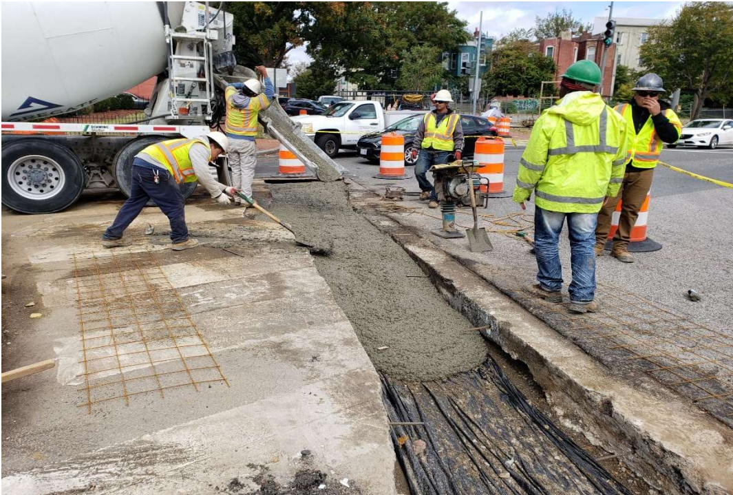
10/17/2019 – PCC Base Construction for utility restoration at 4 th & NY Ave. NE. (North of NY)
