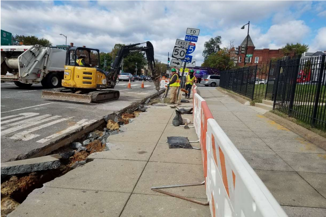
10/17/2019-Demolishing to the old curb/gutter at East side of NJ Ave. b/n Pierce & NY Ave. (North View)
