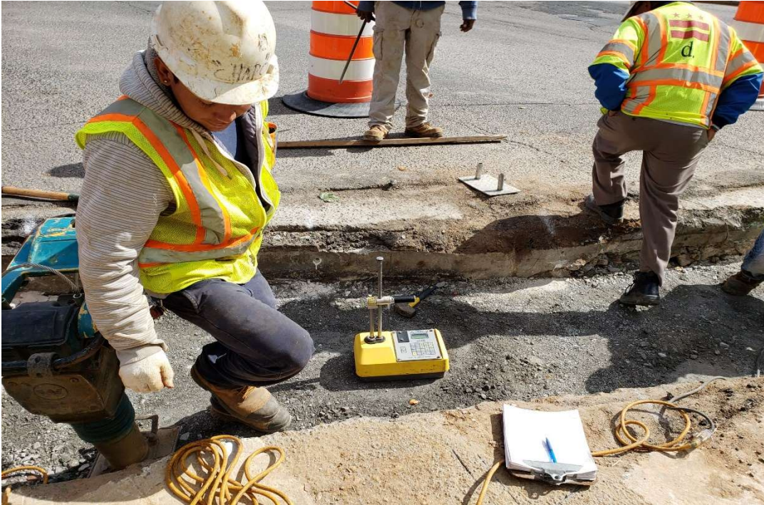
10/17/2019- Moisture-Density test on a soil backfill for utility restoration at 4 th & NY Ave. NW.
