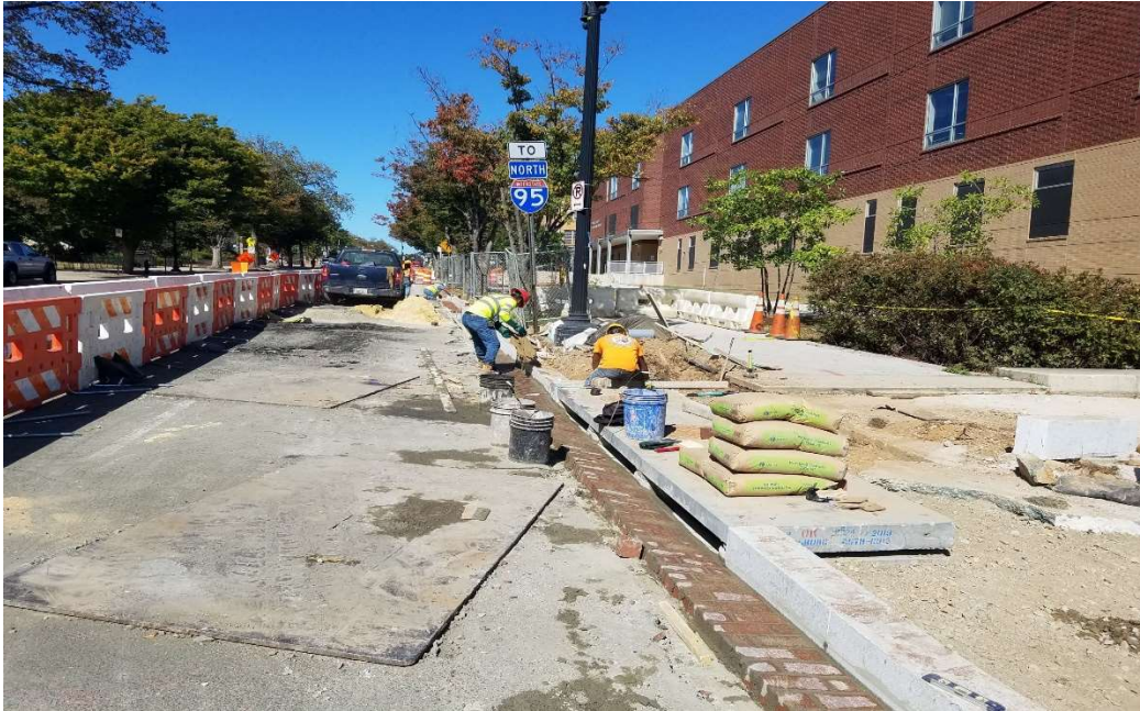
10/14/2019- Brick gutter construction at East side of NJ Ave. NW between L & Pierce St (North View)
