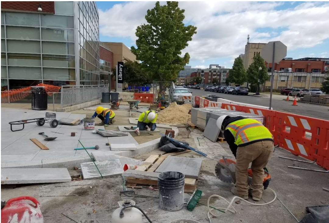
10/17/2019- Block sidewalk construction at NE corner of New Jersey Ave & L St. NW. (East view)
