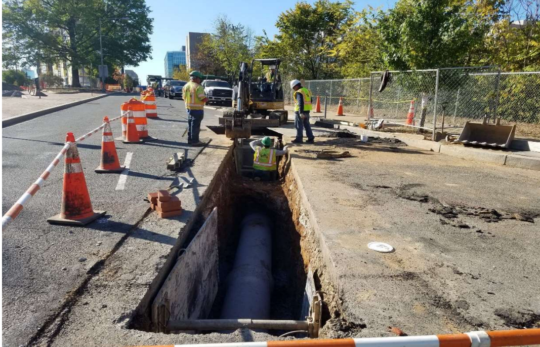
10/15/2019- Installing 18" PCC connect pipes at SW corner of NJ and K St. NW. (South View)
