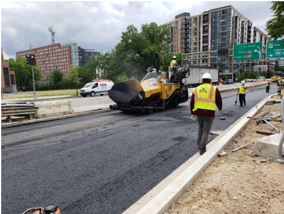
Picture No. 5 – 05/27/2020 – Placed asphalt 25mm base course at NY Ave. between 3rd St. and 4th St. NB. (West View)
