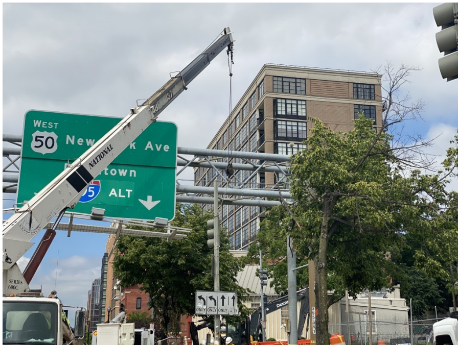
Picture No. 4 – 05/26/2020 – Traffic light transferred at NY Ave. between 3rd. St. and 4th. St
