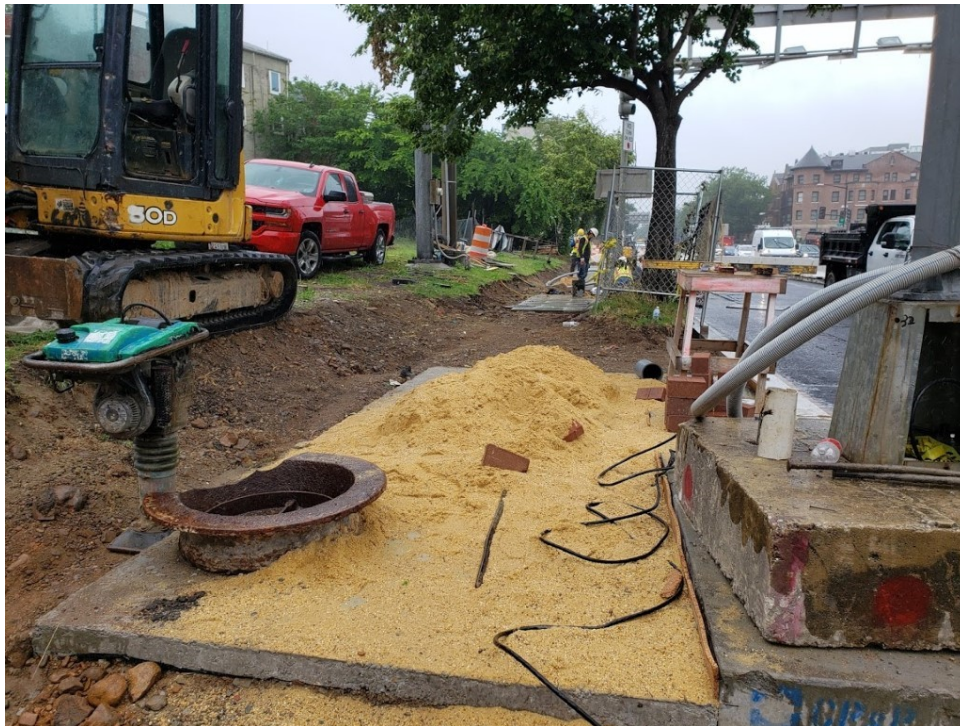
Picture No. 9 – 05/28/2020 – Preparation of the area for sidewalk at NE corner NY Ave. and 4th St. (East View)
