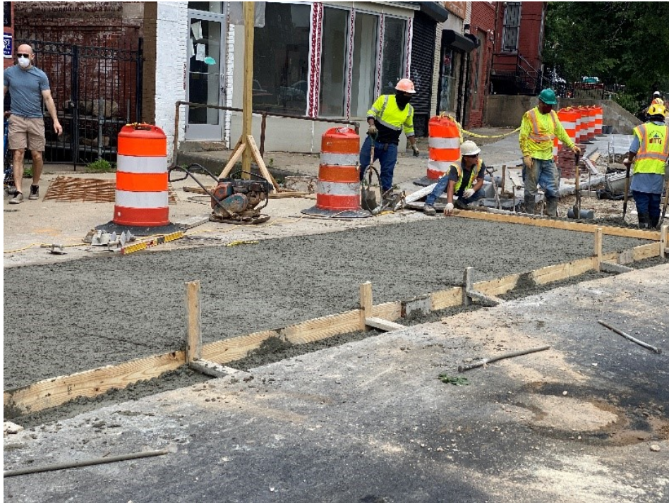
Picture No. 7 – 05/27/2020 –Driveway installation at NY and M St. NW. (East View)
