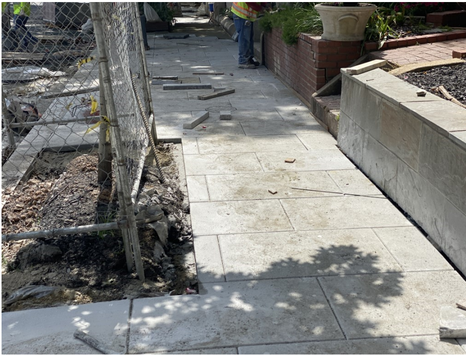
Picture No. 3 - 05/26/2020 – Block Sidewalk on PCC Base at NY Ave. station 310+50 (West View)
