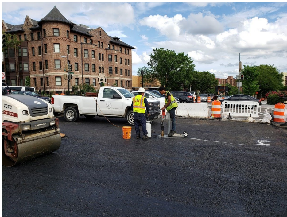
Picture No. 6 – 05/27/2020 – Asphalt coring in progress on the base asphalt paced in the intersection of NY Ave and NJ Ave. (South view)
