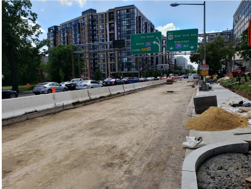
Picture No. 1: 05/26/2020 – Final compaction and grading of aggregate base course underway at NY Ave. between 3rd St. and 4th St. NB. (West View)
