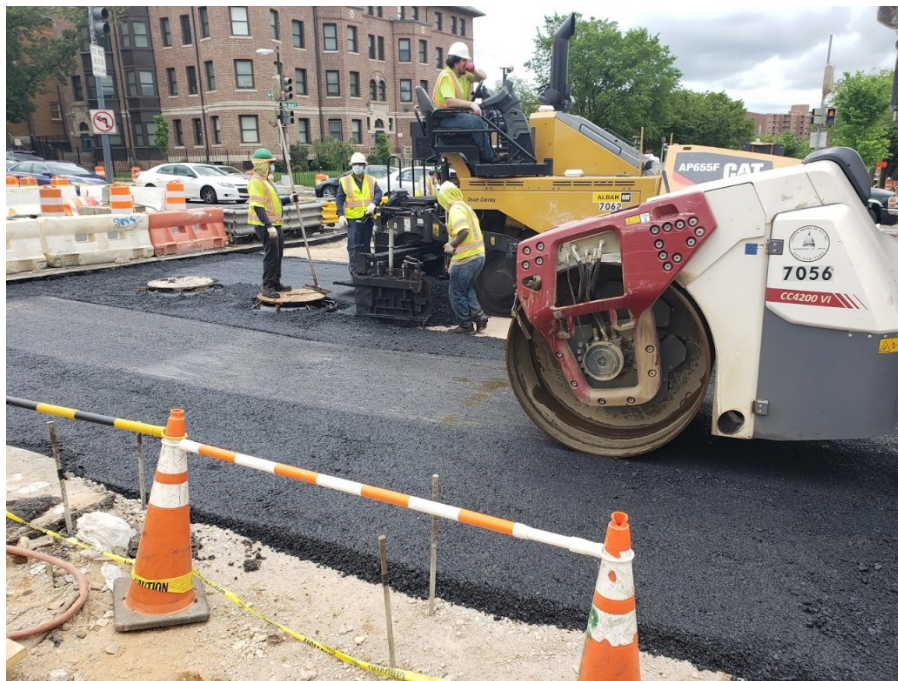
05/27/2020 – Placement and compacting of 25mm base asphalt at the intersection of NY Ave and NJ Ave (South View)
