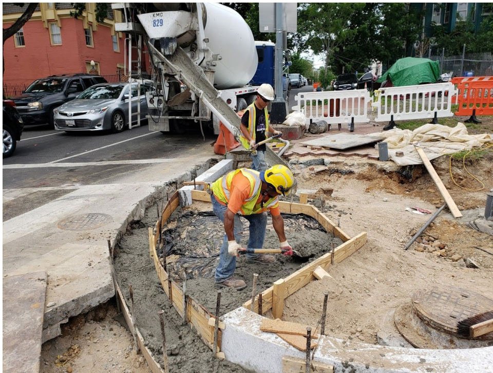
Picture No. 10 – 05/29/2020 – Pouring concrete for gutter base at NE corner NY Ave. and 4th St. (North View)
