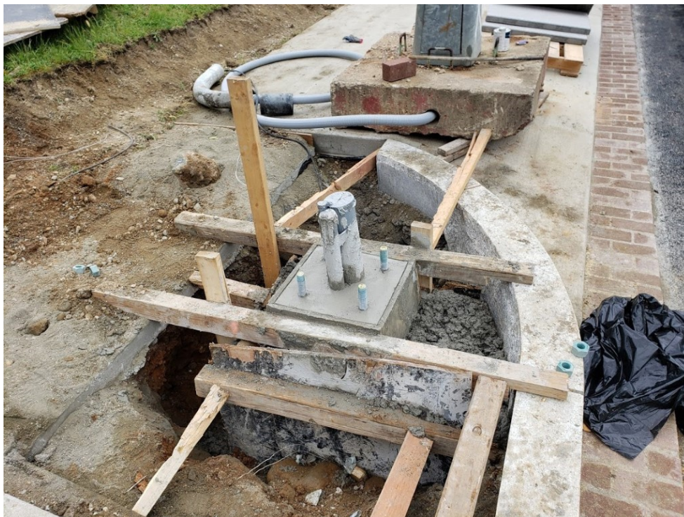
Picture No. 8 – 05/28/2020 – Streetlight foundation PCC work underway at NY Ave. between 3rd St. and 4th St. NB.
